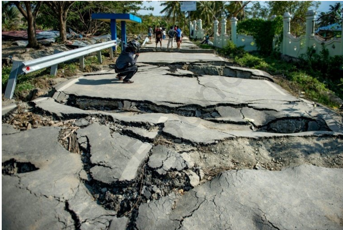
Road damage in Sulawesi
