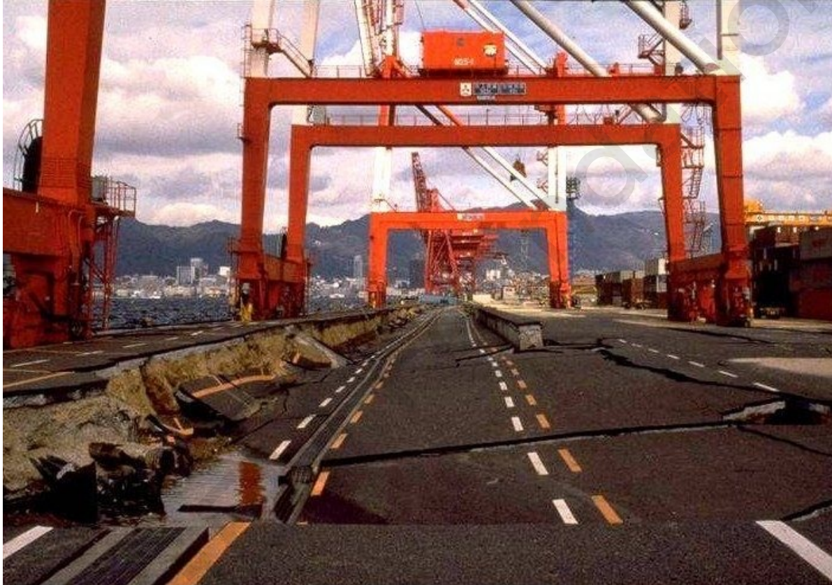
Port damage in Kobe
